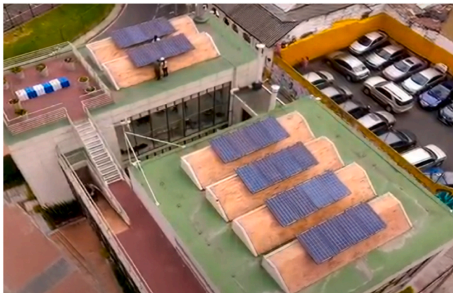
Fig. 9. Photovoltaic system at Universidad Jorge Tadeo Lozano, Bogotá, Colombia.
