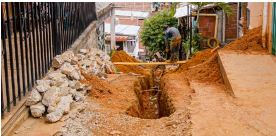
Photographs 8 and 9. Installation of aqueduct and sewerage networks by Emscali Source: Gynna Millán, 2022.
